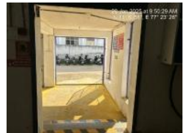
7. Emergency Exit door.JPG
